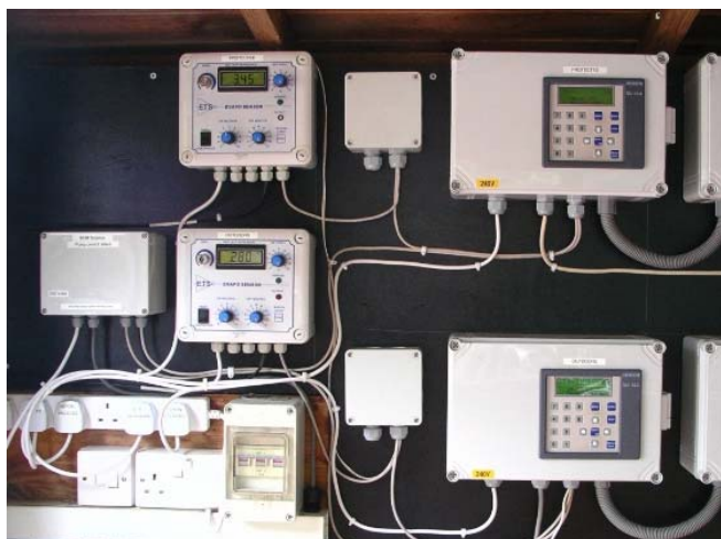
Fig. 3 Two Evaposensor Control Interfaces are here connected to Heron irrigation control panels to achieve automatic 'Evapo-irrigation' scheduling for all the protected and outdoor herbaceous crop beds at W. Godfrey & Sons.
